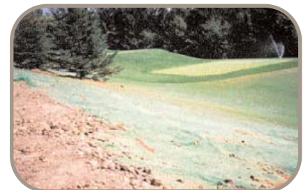
Propex Landlok® SuperGro® was an excellent solution for the potential problems posed by this golf course.
